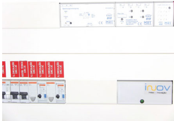
Fig. 5 Energy meters of INOV installed in the electric panel
